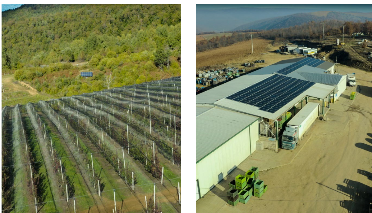
Figure 28 Off-grid solar PV installations: (left) Zajqevc apple tree plantation, and Frutomania processing facility (right)
