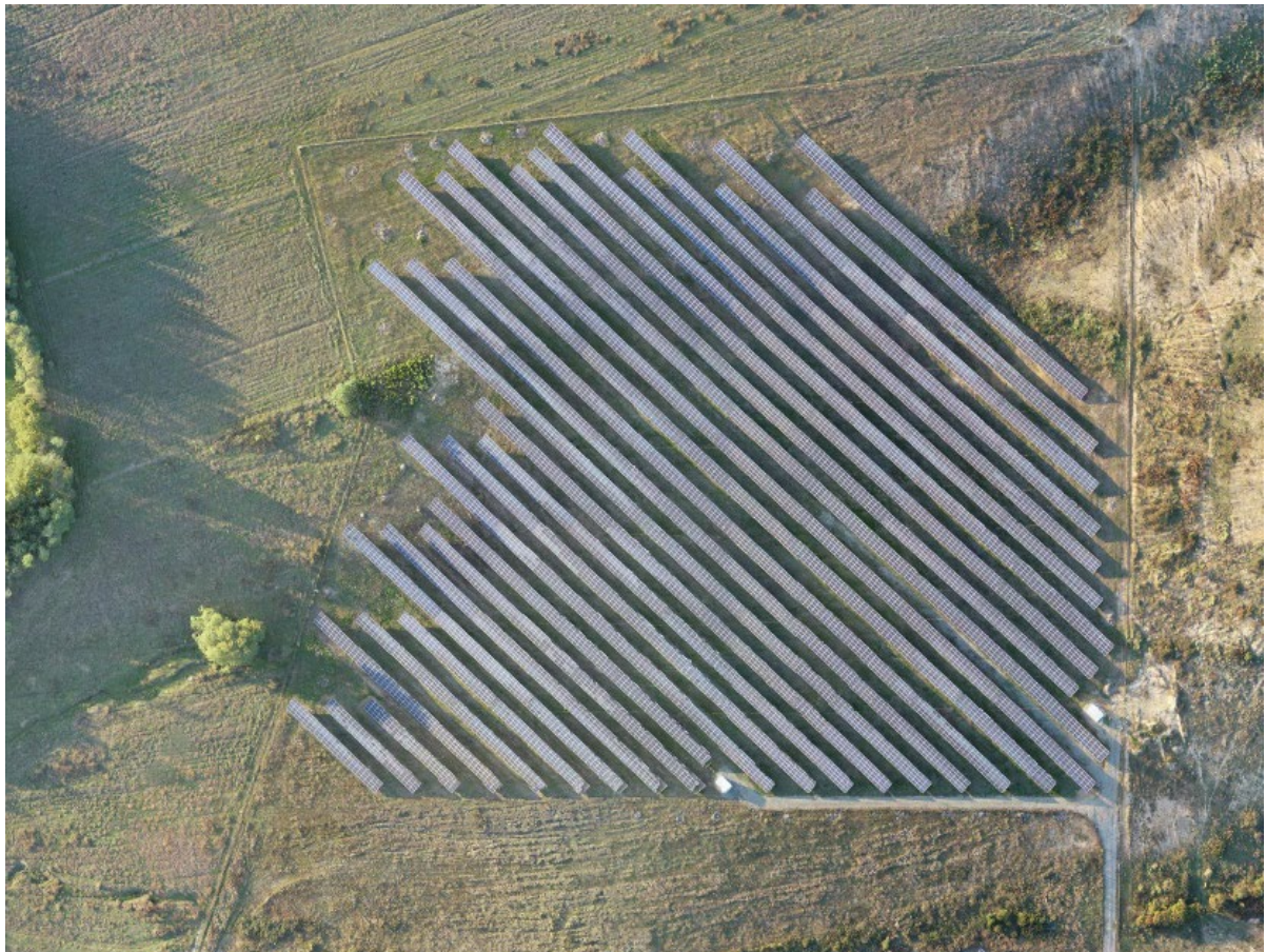
Figure 20 Frigo Food Kosovë, Madanaj-Kusar, Gjakovë, 3,000 kW Solar PV based on Feed-in Tariff
